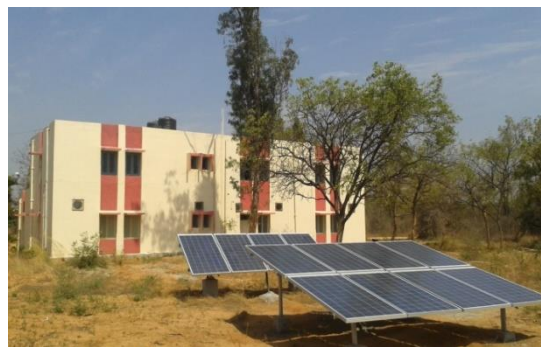
Fig.2.2.1i: Solar power panel set up
